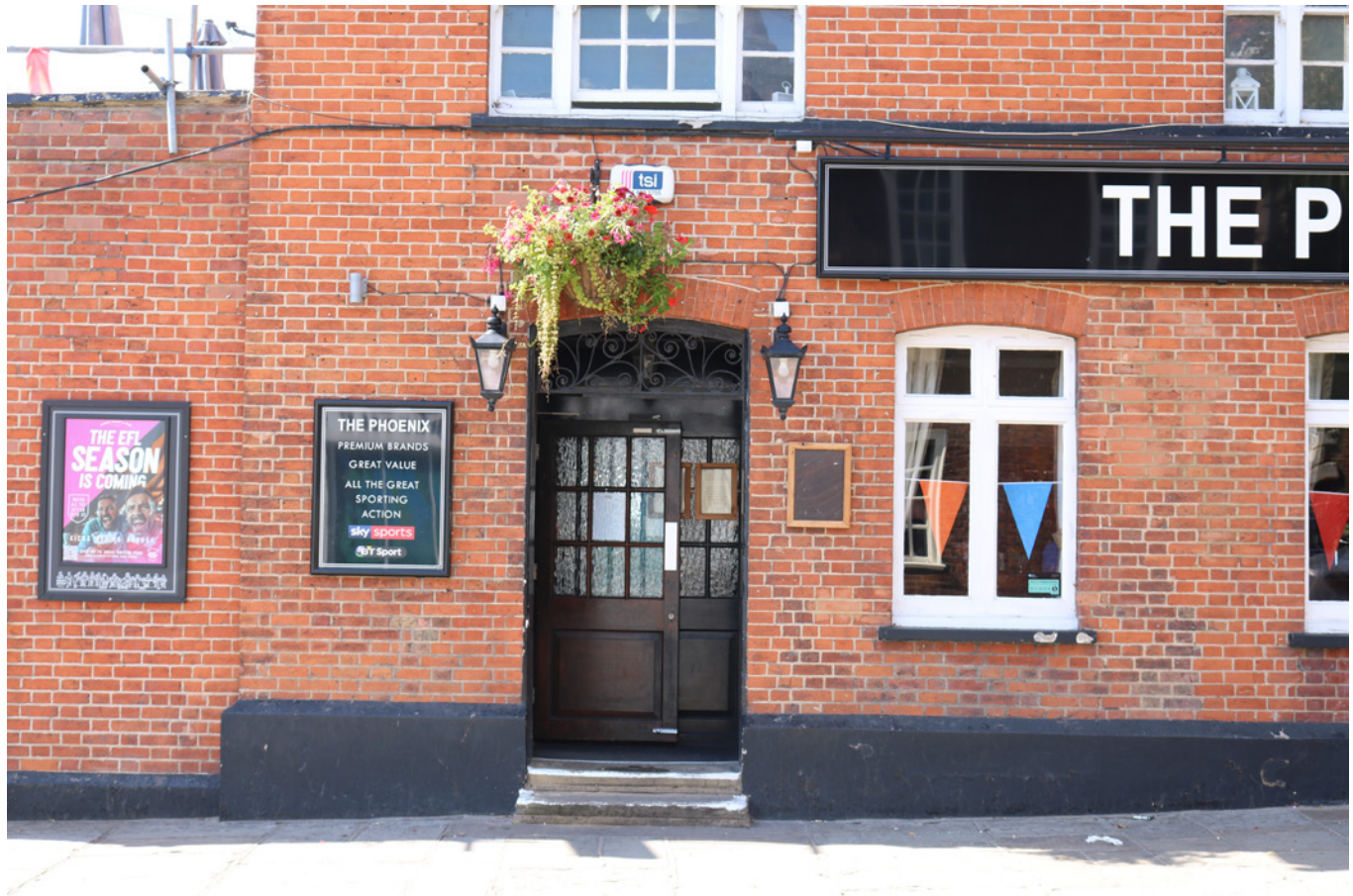
Surface-mounted services & conduit detract from façades
